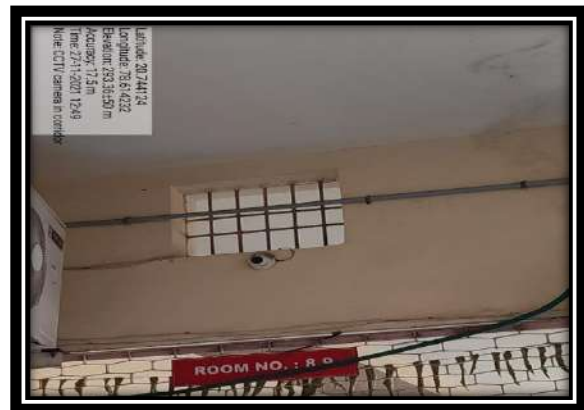
CCTV camera in corridor
