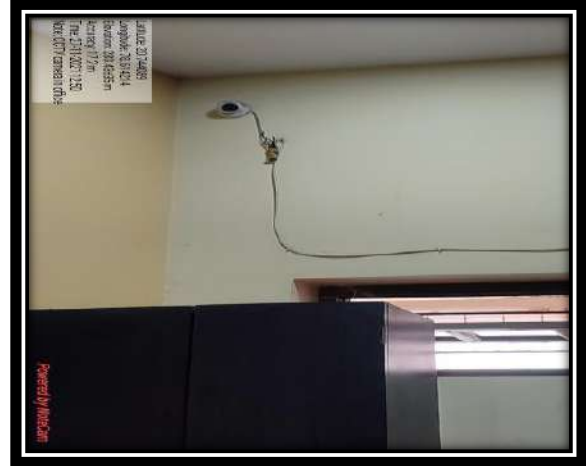
CCTV camera in office
