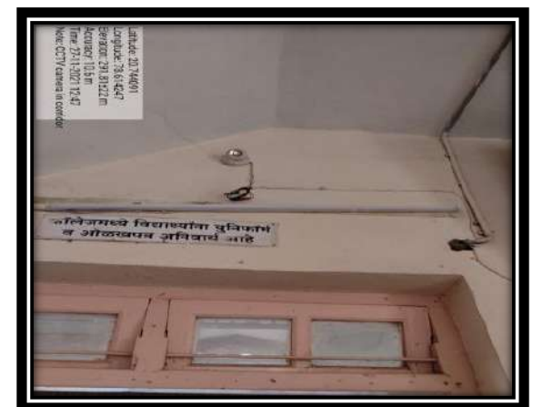
CCTV camera in corridor
