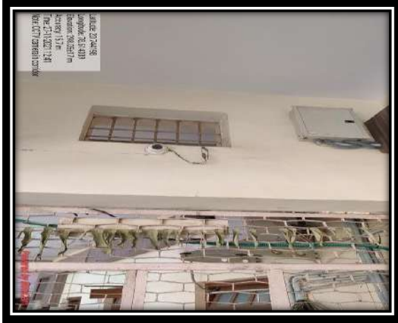
CCTV camera in corridor
